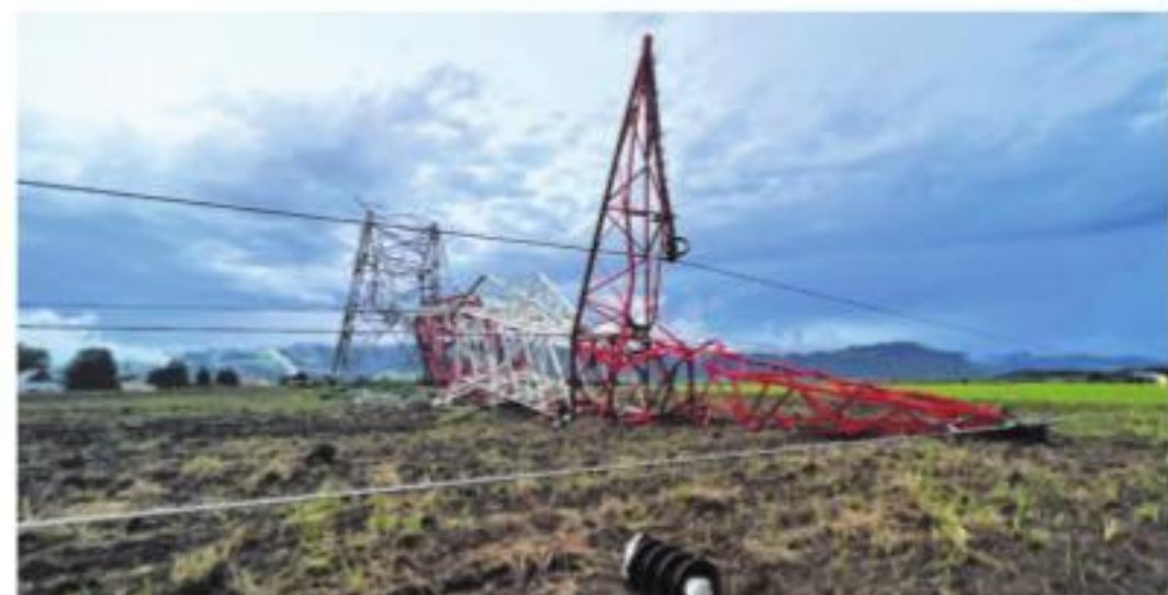
A toppled electricity pylon lying in a field in Styria, south-eastern Austria, after a severe storm hit the Austrian south region on Thursday
